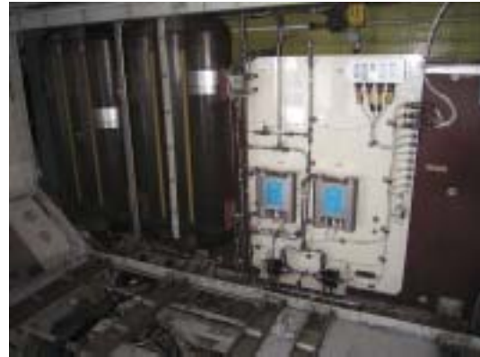
Airbus A310: after C-PWS™ modification to: pumps and water treatment units installed, one tank removed.
